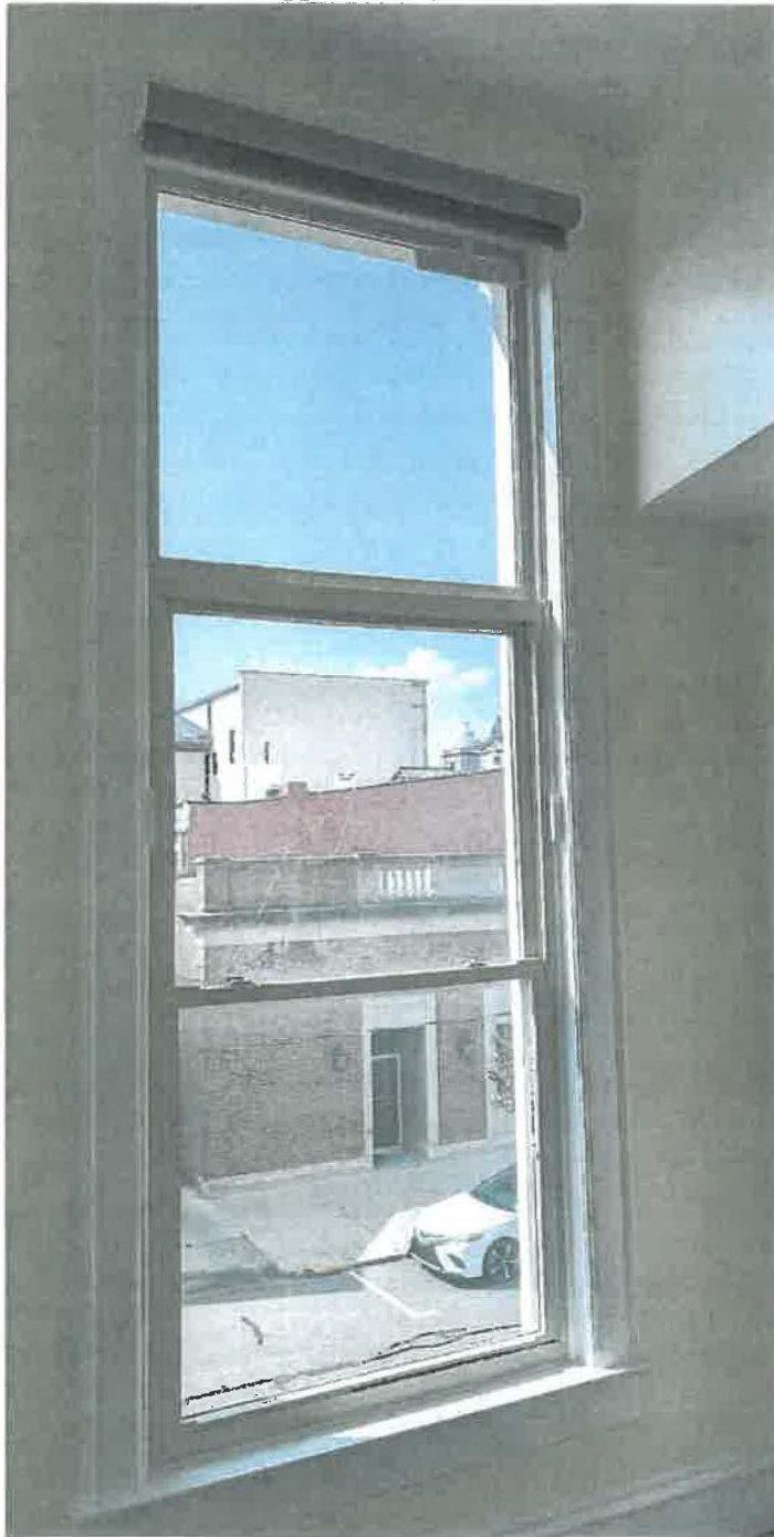
Photo 14: View of triple-pane vinyl design (label: Not Consistent with Original Two-Pane Historic Appearance ).
